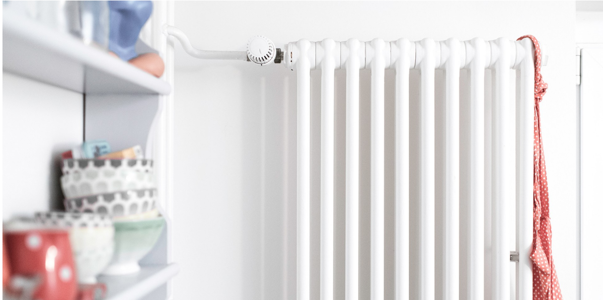
Radiator with thermostat in a Zurich apartment. Source: Christian Beutler Keystone
