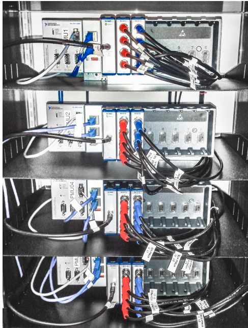
Demonstration of real-time control of electricity flows in the real microgrid of the EPF Lausanne. Source: Project “ Real-time control of power flows ”
