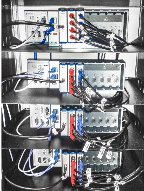
Demonstration of real-time control of electricity flows in the real microgrid of the EPF Lausanne. Source: Project “ Real-time control of power flows ”
