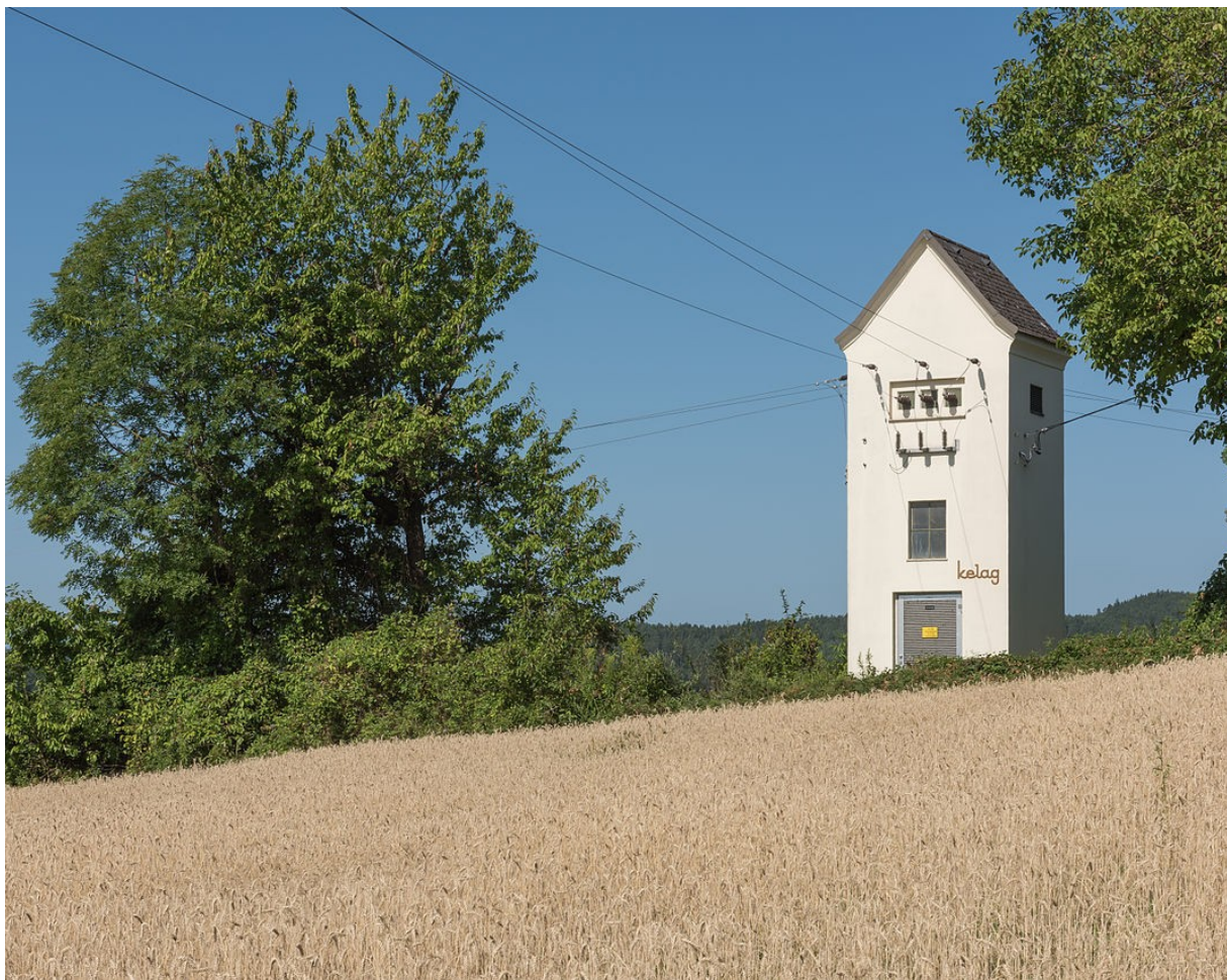
In transformer stations, transformers are used to switch electrical current from one voltage to another. Source: Wikimedia Commons
