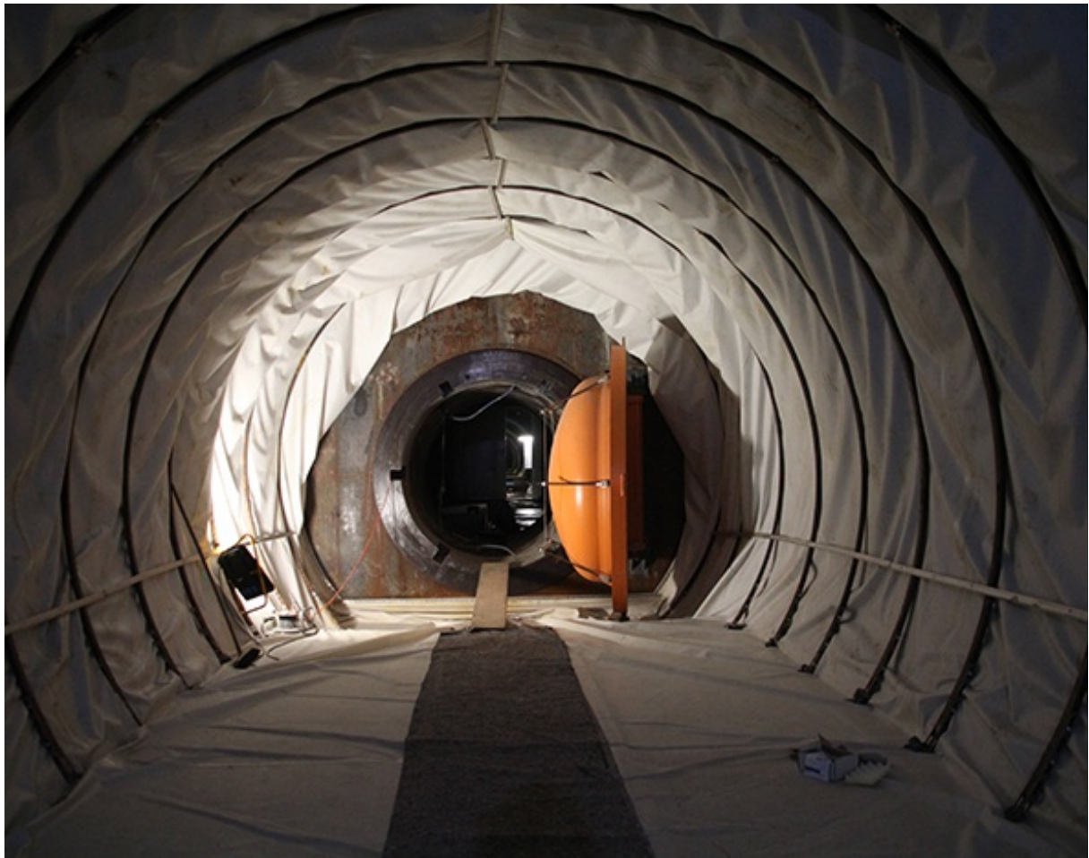
The inside of a compressed air reservoir – here, compressed air is stored in the mountain. Source: ALACAES
