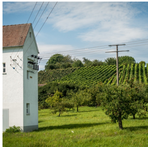
SiC solid-state transformer in the grid
