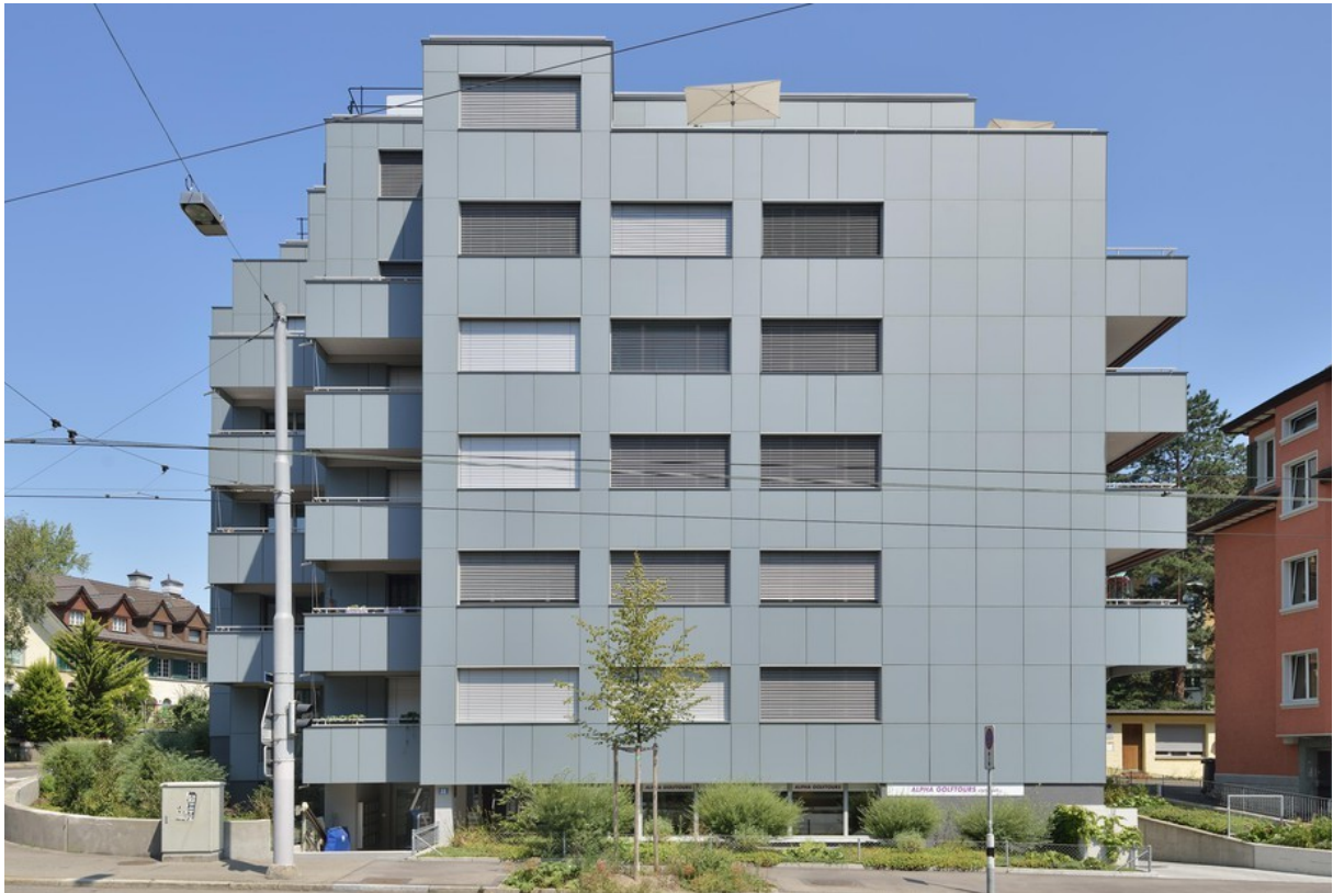
A plain Jane? Far from it – photovoltaic modules are integrated in the facade of this multi-family dwelling in Zurich. Source: O. Wavre / LAST / EPFL
