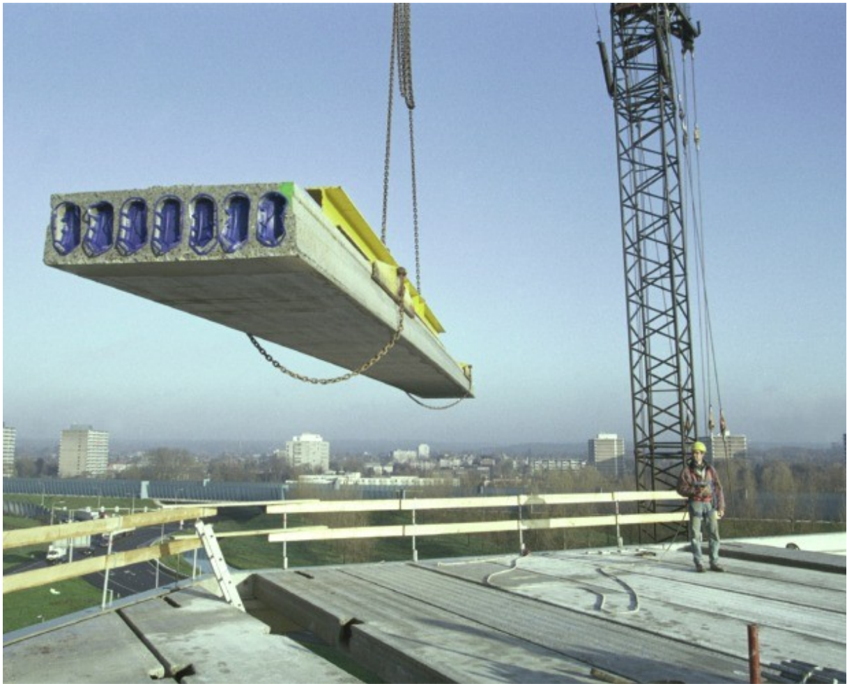
As the name suggests, prestressed concrete is prestressed, giving it greater tensile strength. Source: Wikicommons/Michael Schmahl
