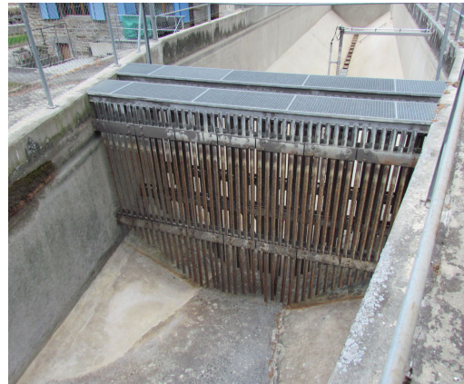
Rakes in the basins calm the water flow and contribute to efficient desanding. VAW / ETHZ
