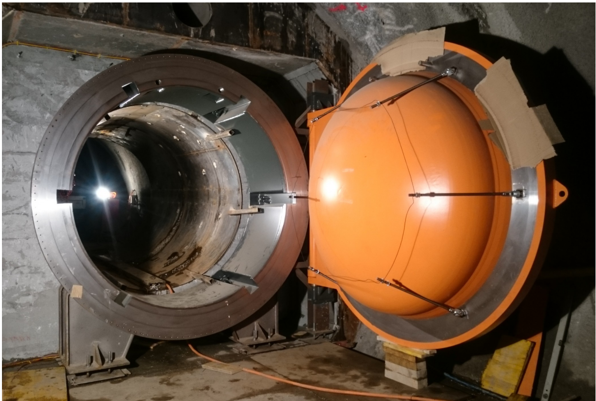
A compressed air reservoir in the Alps: the storage of electricity generated from renewable sources is being tested here. Source: ALACAES
